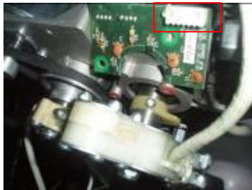
1 terminals on the board
