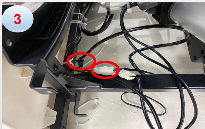
d. disconnected the terminals
