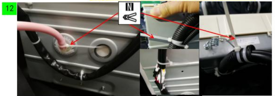
The cable ties was tied to the back line and trachea, cut the tail end of cable ties off with diagonal cutter.
