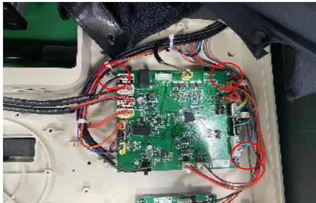
D.discontent the terminals and screws
