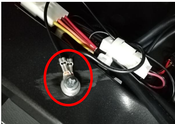
Nine-core connecting wire and 32 core wire earth wire with lock
