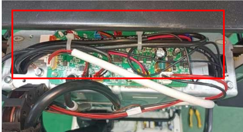
Disconnect the signal terminal
