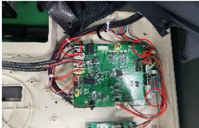
D.discontent the terminals and screws
