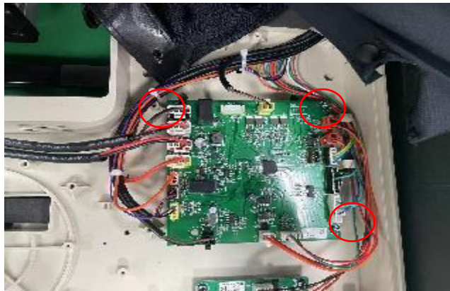
D.discontent the terminals and screws
