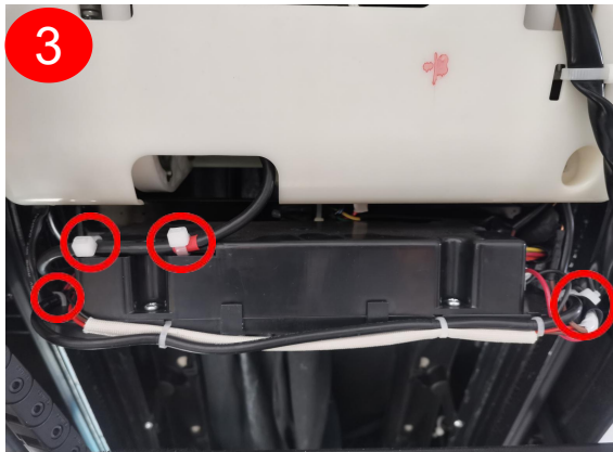
cut cable tie
