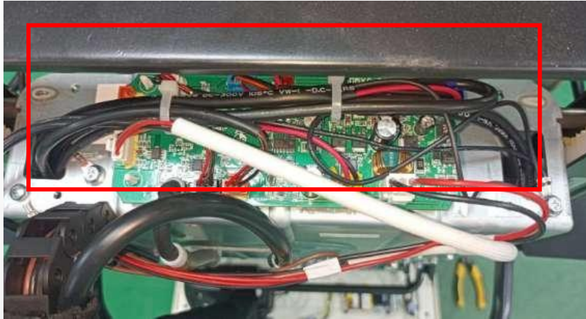
Disconnect the signal terminal
